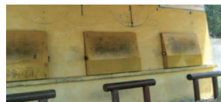
Holes in walls
